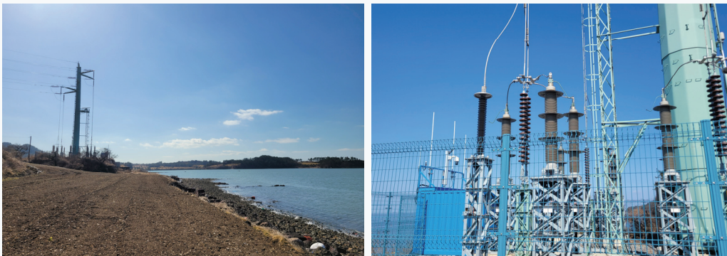
Landfall point of the Subsea Transmission Line in Mokpo
