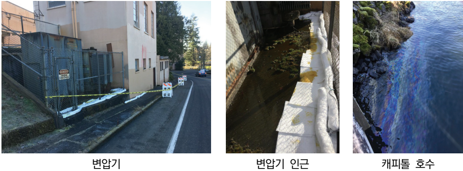
자료: Flickr(2019.2), "Olympia Brewery Transformer Spill", 검색일: 2024.9.1.
